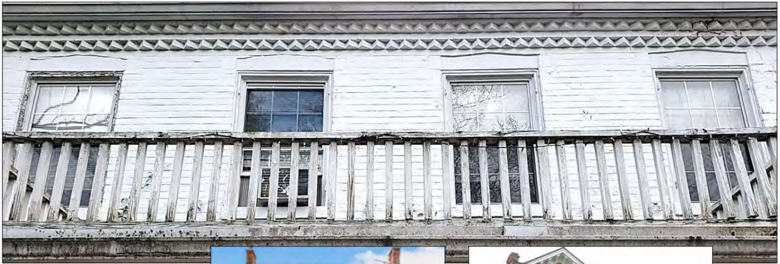
Inconsistent Window Headers
